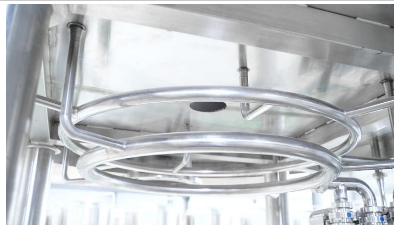
Ring pipe for collecting wort and backwash on bottom
